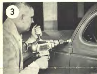
Put drill bushing in outside bracket and drill hole with 1/2" drill. The angle is pre-determined by bracket and drill bushing. Hold drill level.
